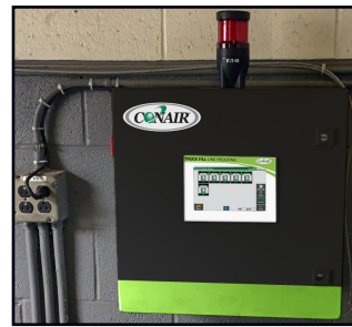
Truck Fill Proofing Control
