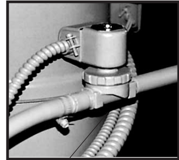
Typical make-up solenoid valve Figure 3.2A
