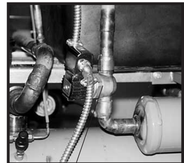
Typical liquid line solenoid valve
