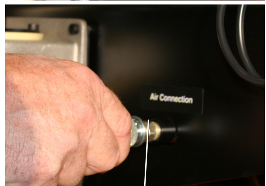
Air Hose Connection
