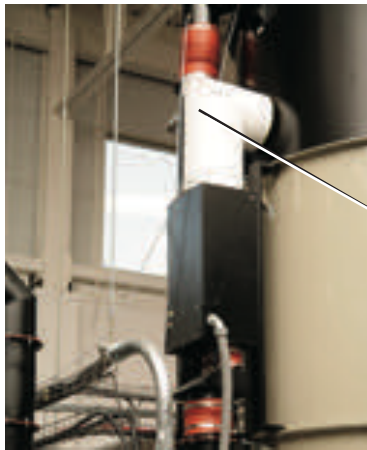
HTC Outlet to CH Hopper Inlet Connection
